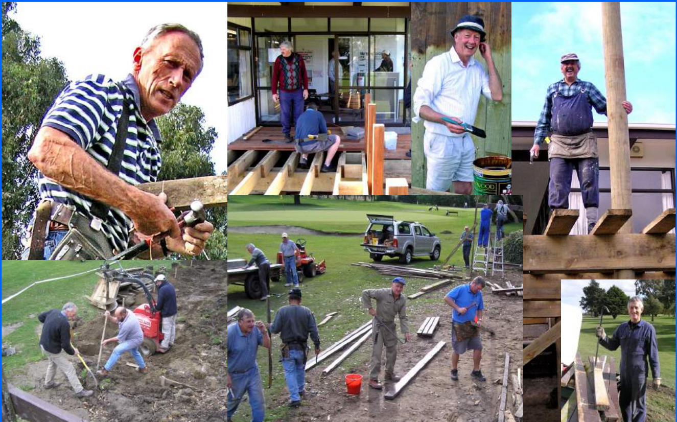
Snaps during construction of the new balcony: (Ray Richardson, Master Builder at top left)
